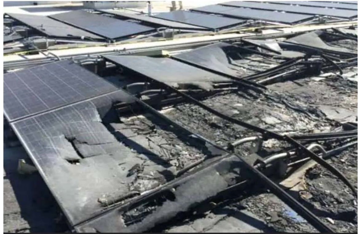
Walmart roof fire, USA
