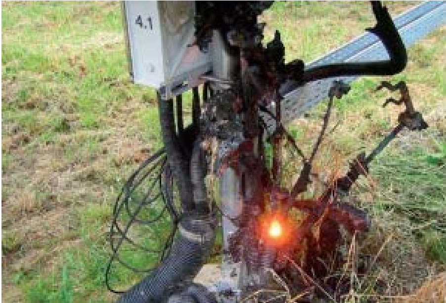
Glowing arc fault in the dc wiring at the combiner box
