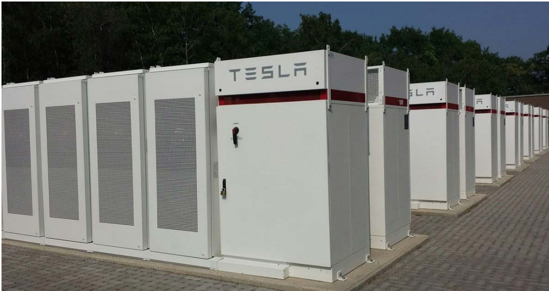
18 MW battery units by Tesla (Dilsem-Stokkem)
