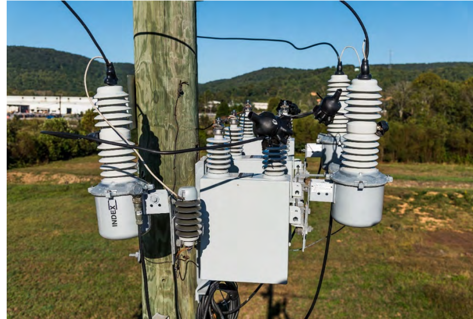
Capacitor bank, faulty switch on front right
